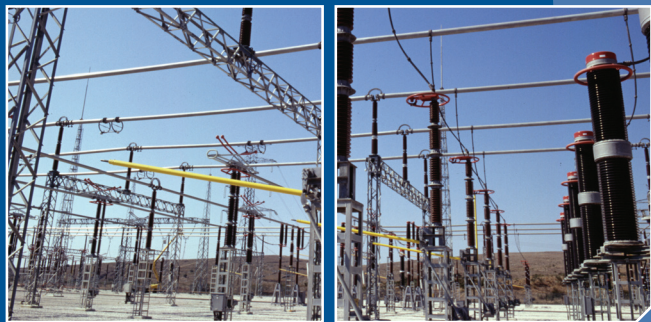
Power Systems Automation
